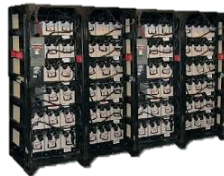
Battery Inc. in UPS Losses
